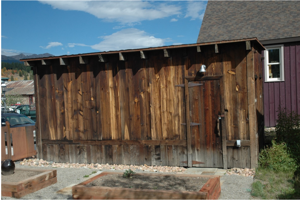
CD 1, Image 80, View to North, of the south-facing wall of the shed
