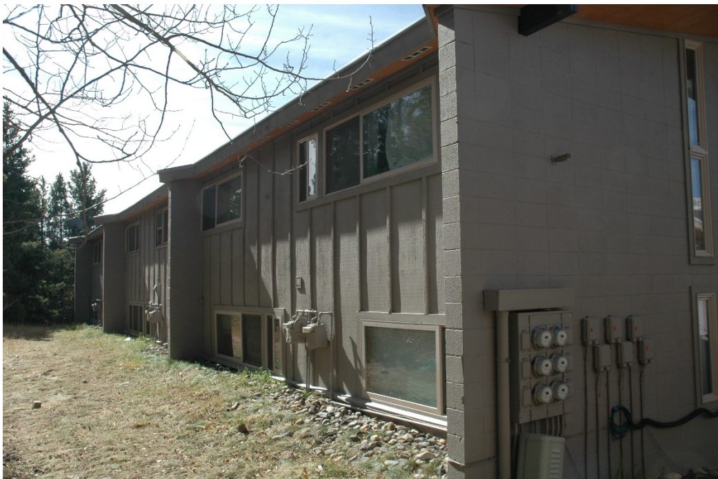
CD 1, Image 37, View to Southwest, of the east end of the north-facing wall and the east-facing wall of the south building.
