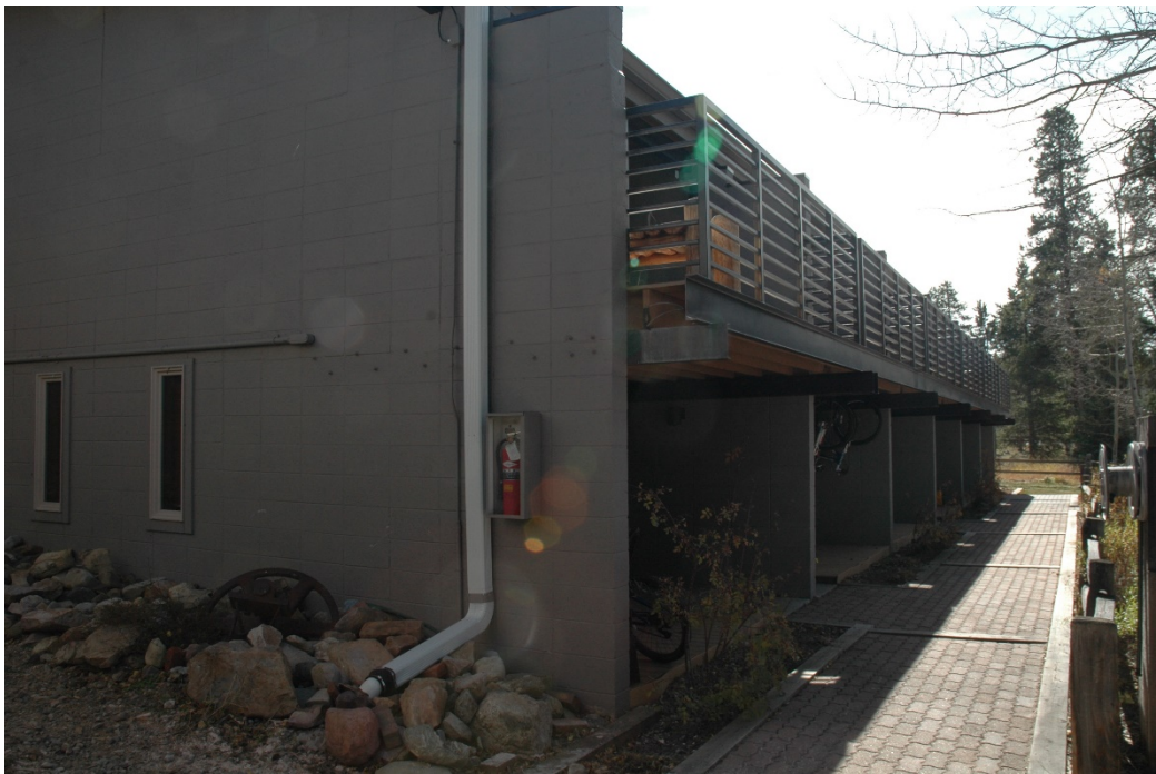
CD 1, Image 31, View to Southeast, of west-facing and north-facing walls of the south building.
