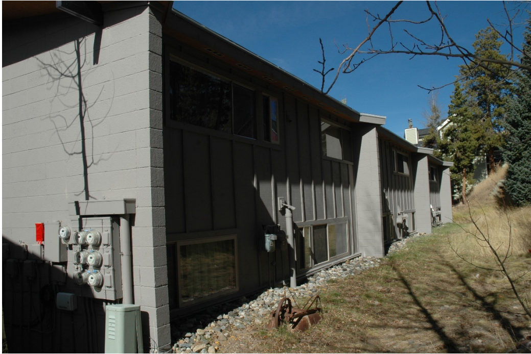
CD 1, Image 38, View to Northwest of the east end of the south-facing wall and the east-facing wall of the north building.
