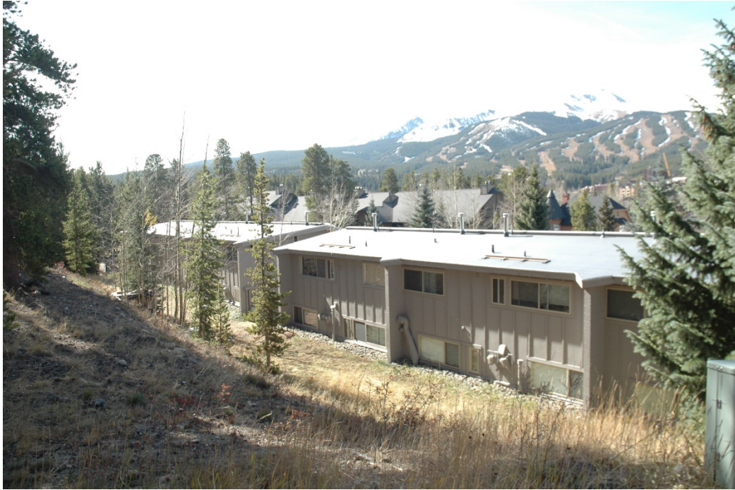
CD 1, Image 40, View to Southwest, of the east-facing walls of both buildings.
