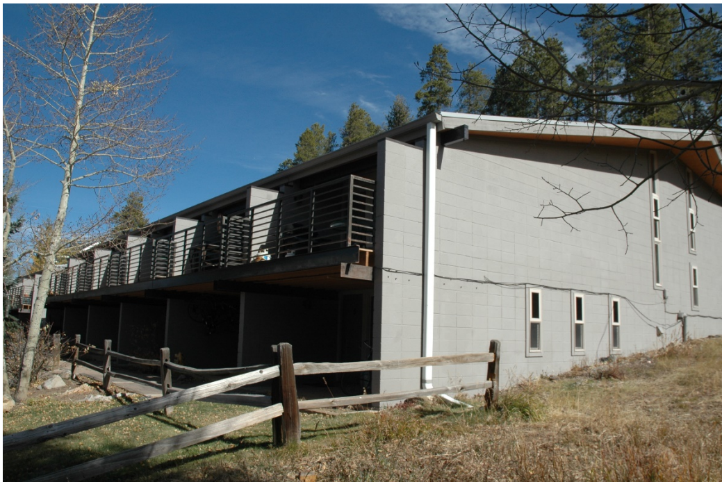
CD 1, Image 33, View to Northeast, of west-facing and south-facing walls of the south building.
