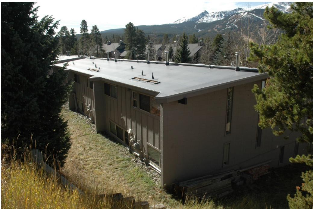
CD 1, Image 39, View to Southwest, of the east-facing and north-facing walls, and the roof of the north building.
