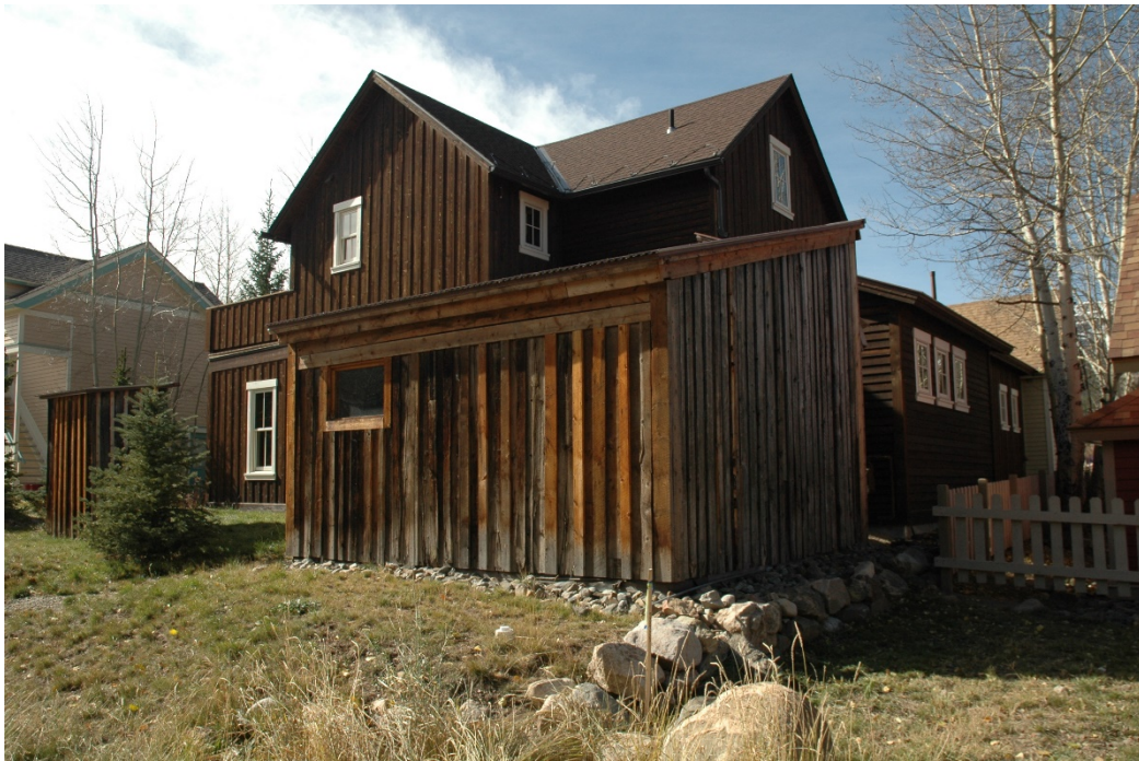
CD 1, Image 11, View to Southwest, of the shed and privy, and of portions of the east-facing and north-facing walls of the addition.
