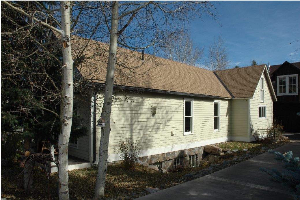
CD 1, Image 8, View to Northeast, of the south-facing wall of the original dwelling.
